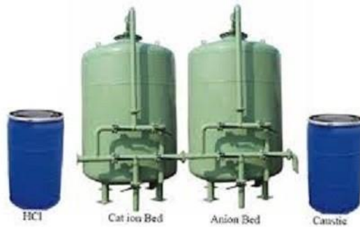
Gambar IV.A.3 Demin Water Plant
